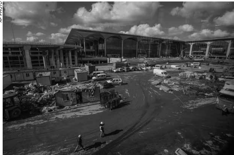
Construction continued last week in Istanbul's new airport ahead of its opening
