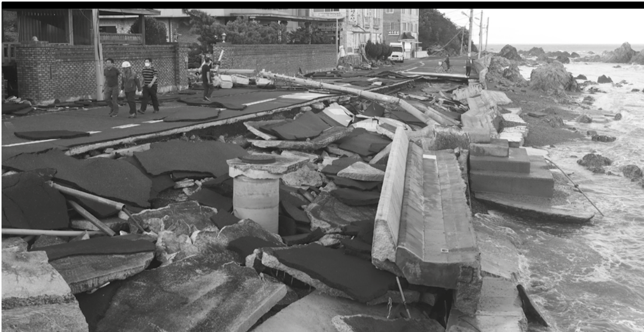
A coastal road is damaged in Ulsan, South Korea
