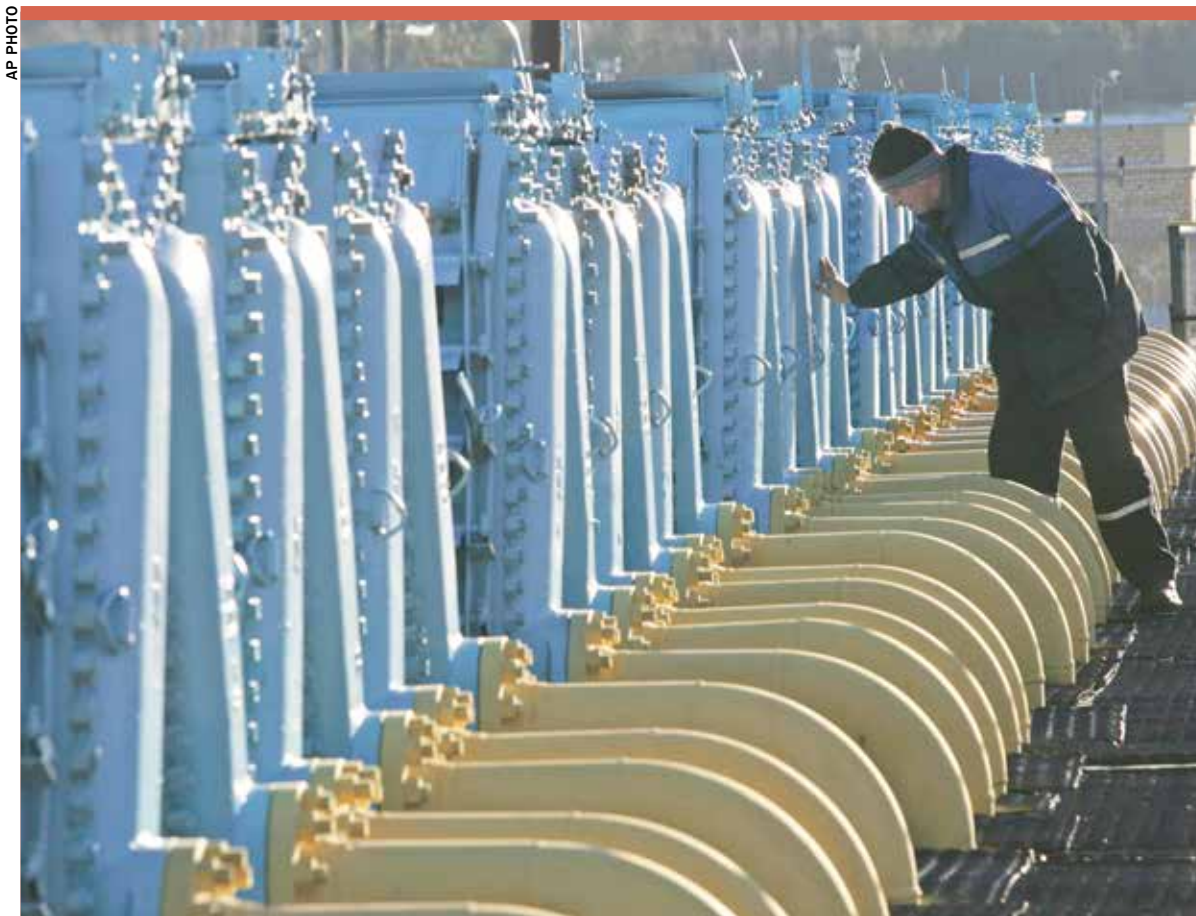
A gas compressor station of the Yamal-Europe pipeline near Nesvizh, some 130 km southwest of Minsk, Belarus
