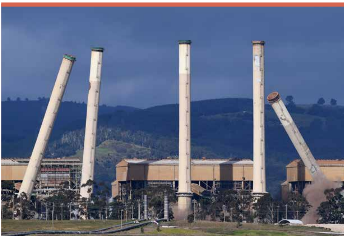
Some of the coal-burning Hazelwood Power Station's eight chimneys begin to topple as they are demolished and the station is decommissioned in Hazelwood, Victoria
