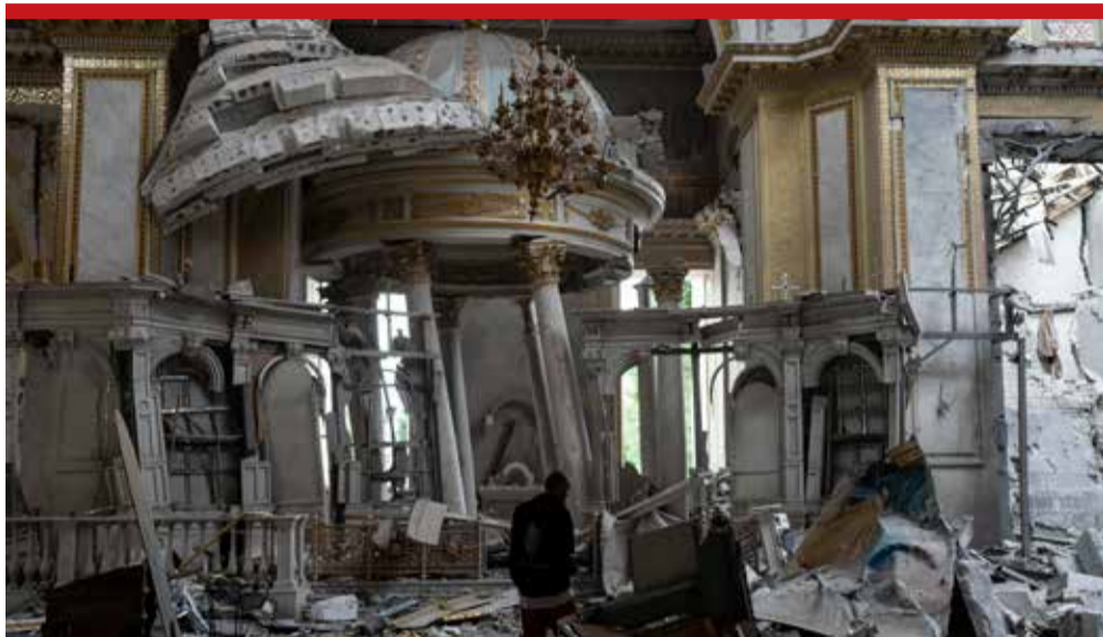
A church personnel inspects damages inside the Odesa Transfiguration Cathedral in Ukraine
