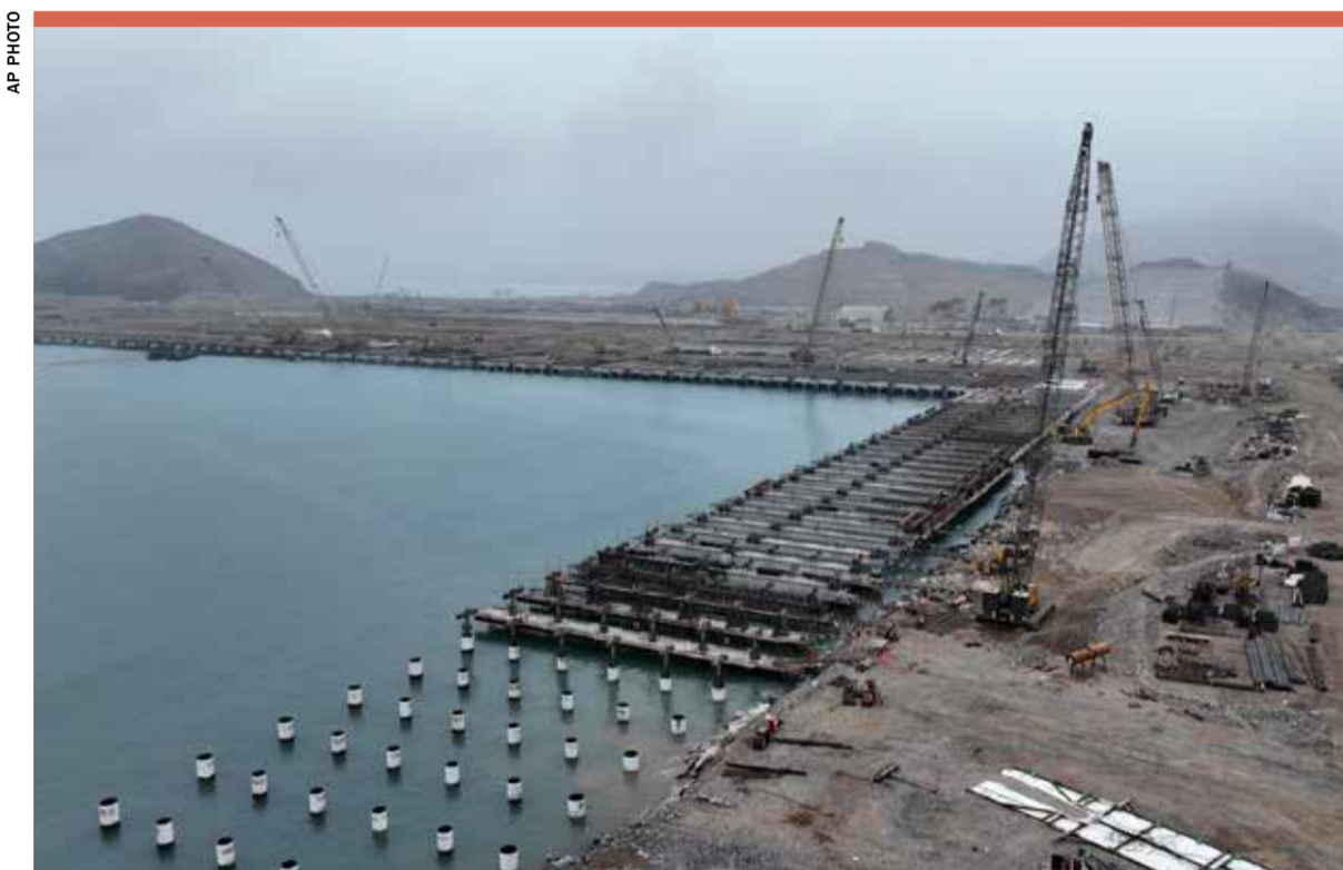
Cranes work in the construction of the Chancay Multipurpose Port Terminal, built by a Chinese company in Chancay, Peru
