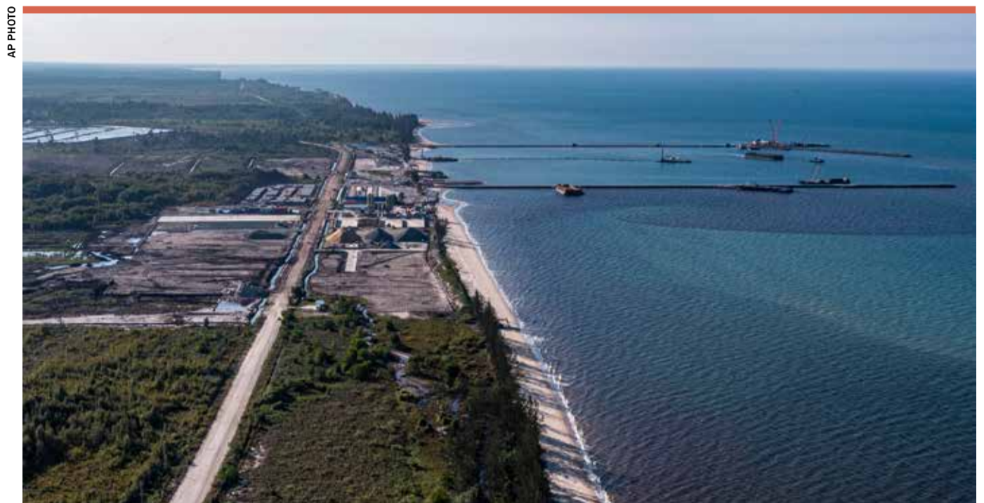
The construction site of the Kalimantan Industrial Park Indonesia (KIPI) is visible in Mangkupadi, North Kalimantan
