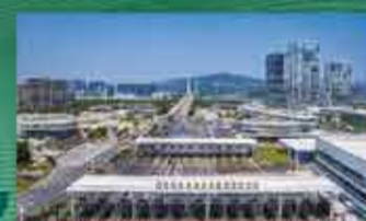
The customs supervision sites and supporting facilities at the 'second-line' places are under construction
