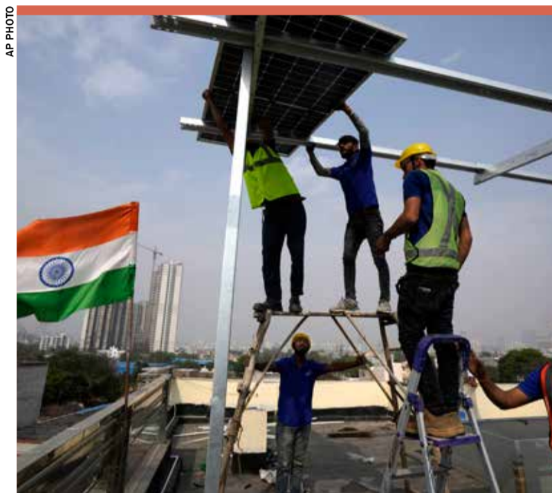
Workers of Solar Square place a panel on the rooftop of a residence in Gurugram on the outskirts of New Delhi
