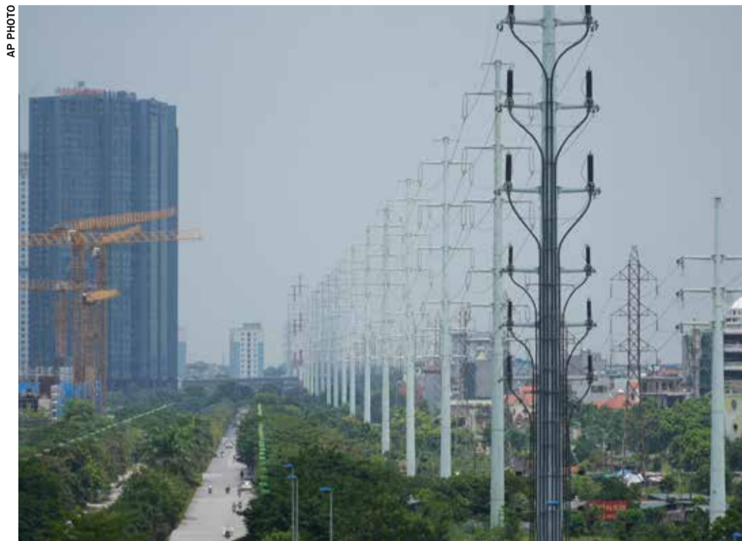
Power lines in Hanoi
