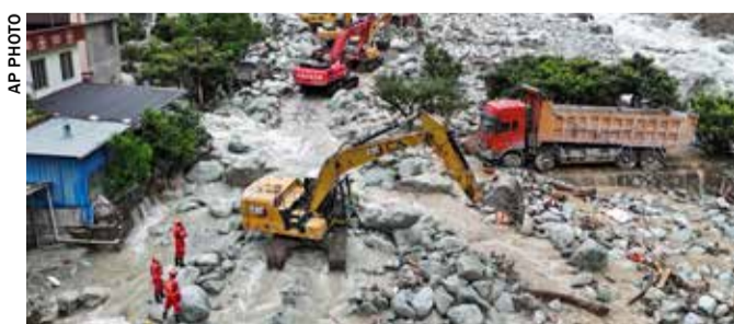
Rescuers operate excavators to restore access on National Highway 318 in the aftermath of flash floods and mudslides in Ridi Village, Kangding City, Garze Tibetan Autonomous Prefecture
